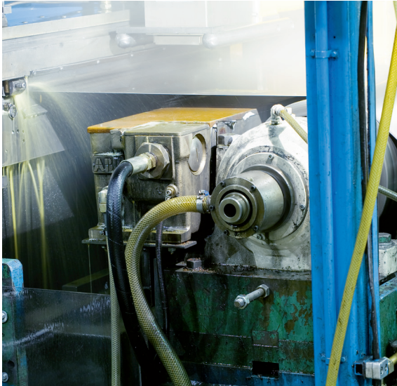
Stressometer Flatness Control System combined with Millmate Strip Scanner in a reversible cold mill.
