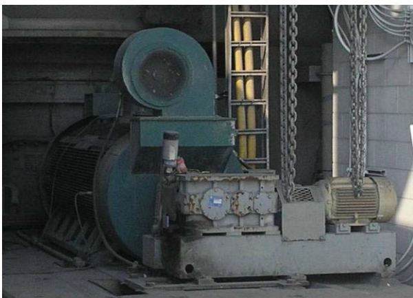
Figure 6: Inching Drive on NDE of Mill Drive Motor
