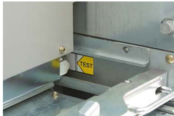
Circuit breaker in TEST position
