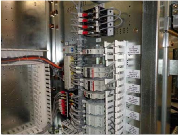
Heater load terminals in low voltage compartment (typ.)
