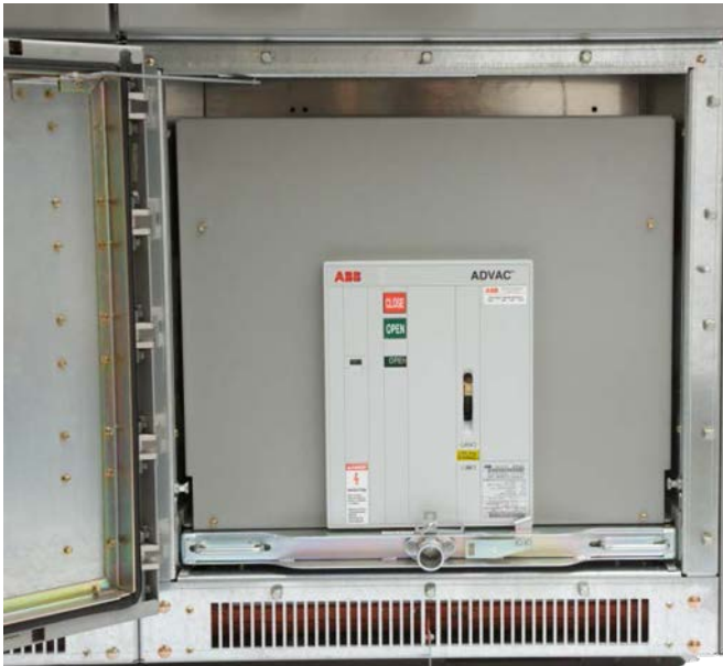
Circuit breaker in DISCONNECT position
