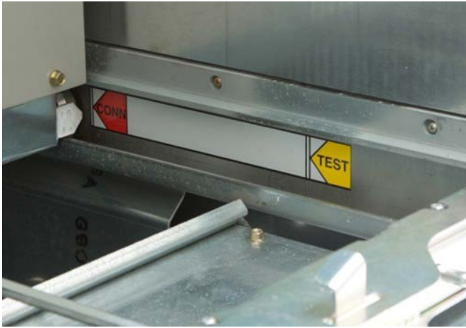
Circuit breaker in CONNECTED position
