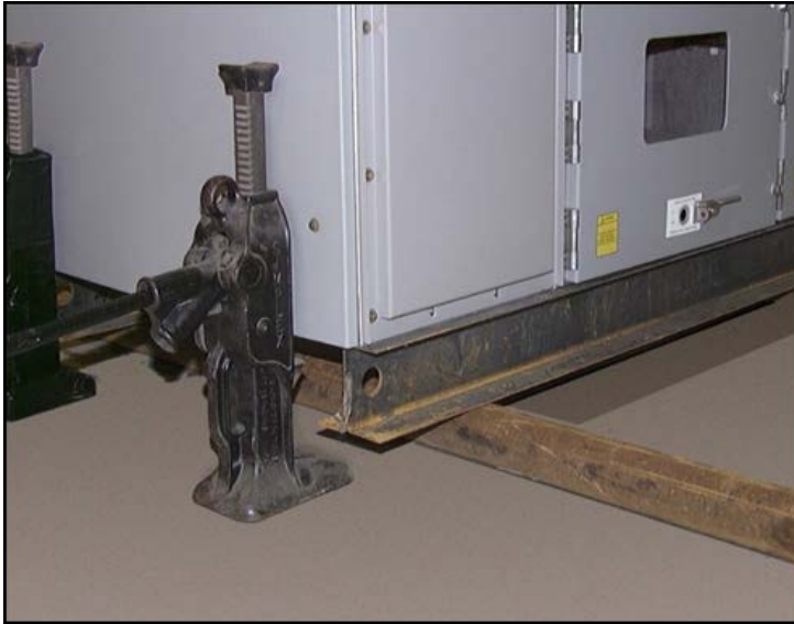
Placement of jacks at the corners with rollers under the shipping bases
