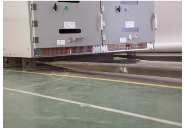
Forklift forks penetrating shipping channels
