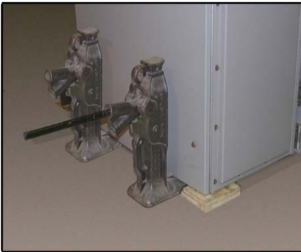
Jacks lower the frames onto wood blocks a pry bar to remove the wood blocks
